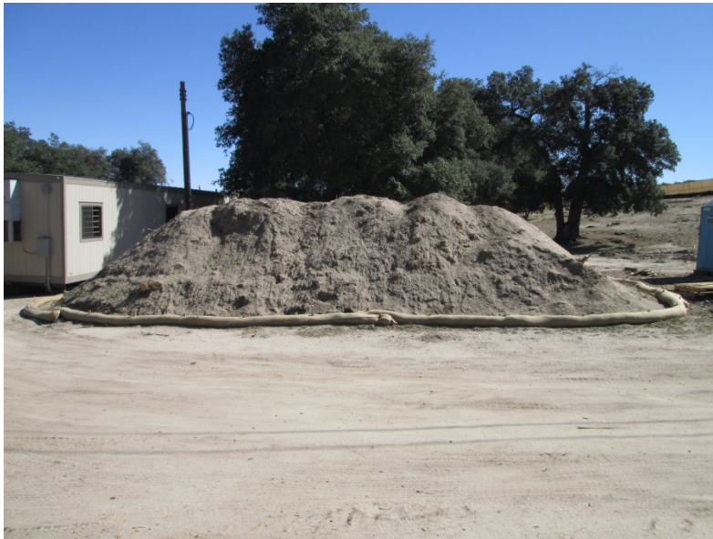
Photo 2: In accordance with Mitigation Measure BIO-1D, topsoil is being salvaged for future restoration efforts at the Boulevard Rebuild Substation.
