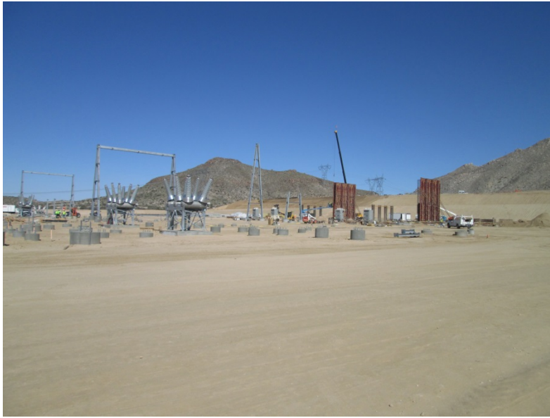
Photo 5: Construction activities associated with foundation drilling, concrete form building and firewall construction continue at the ECO Substation pad site.
