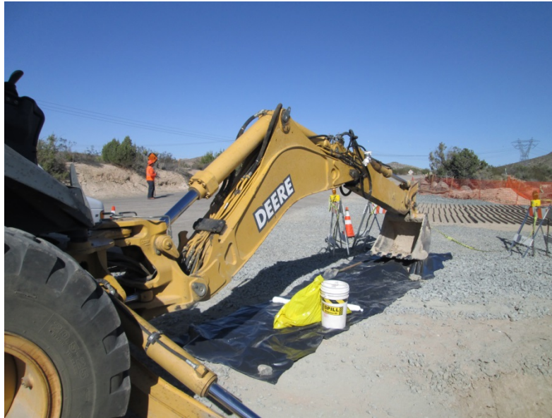
Photo 3: Spill kits are utilized during construction to manage hazardous materials in accordance with Mitigation Measures HAZ-1a.
