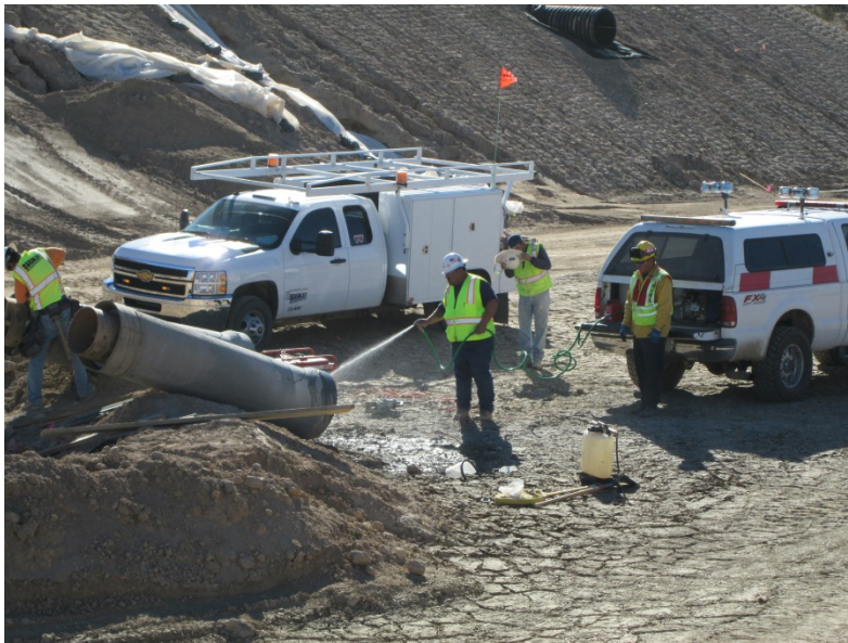
Photo 6: In accordance with the Construction Fire Prevention Plan (Mitigation Measure FF-1), a fire watch waters down concrete piping following cutting activities at the ECO substation pad.
