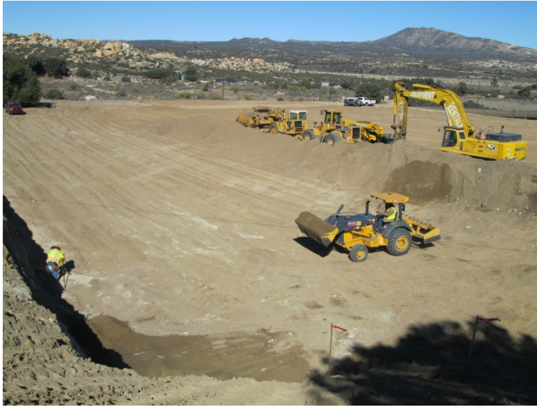
Photo 1: Construction activities continued at the Boulevard Rebuild Substation consisting of rough-grading the substation pad.
