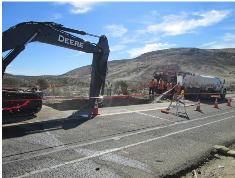
Photo 4: Construction activities associated with vault excavations for the 138 kV Underground Transmission Line component were completed along Old Highway 80 during this reporting period. A water truck is utilized to reduce fugitive dust emissions in accordance with Mitigation Measure 4a and the Dust Control Plan.
